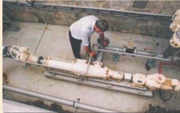
RM681 Pump in Waste Water Treatment Plant at Auckland (New Zealand)
