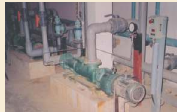
RD551 Pumps for Degremont Plant at Delhi (India)
