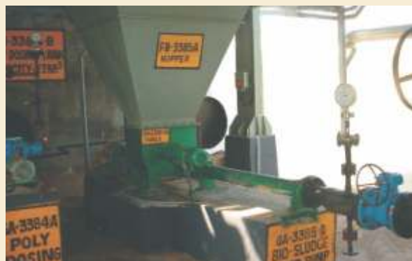
KM584 Pump with Bridge breaker feeding incinerator at Reliance, Hazira (India)
