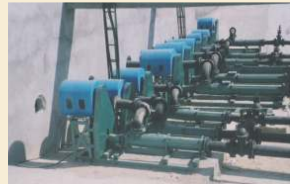
Battery of RL Series Pumps for Tannery Effluent at Unnao Banthar (India)
