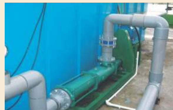
RM621 Pump in Waste Water Treatment Plant at Malaysia
