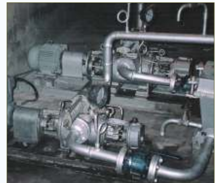
Twin Screw Pump pumping resins at a facility in Kolkata, India
