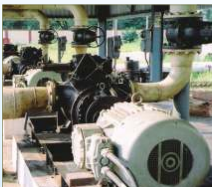
Twin Screw Pump pumping Carbon Black Feed Stock at a facility in Egypt
