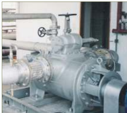
Twin Screw Pump pumping Chemical at a facility in Malaysia
