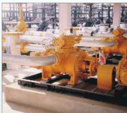
Twin Screw Pump pumping Kerosene Oil at a facility IOCL Balasore Terminal, India
