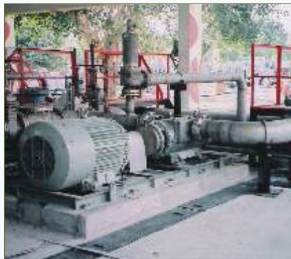
Twin Screw Pump pumping Aviation Turbine Fuel at a facility Indian Air Force Agra, India
