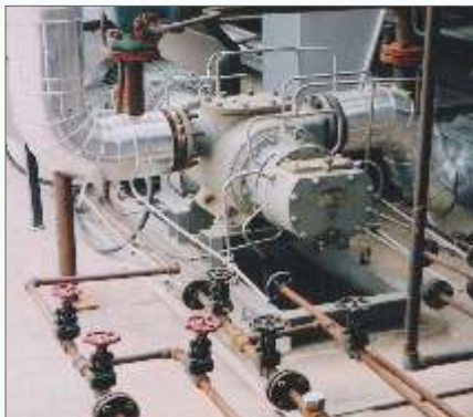
Jacketed Twin Screw Pump pumping Bitumen (C.R.M.B) at a facility IOCL Mathura Terminal, India
