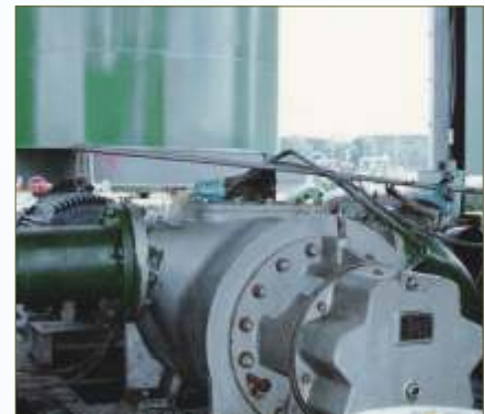
Twin Screw Pump pumping Molasses at a facility in Vietnam
